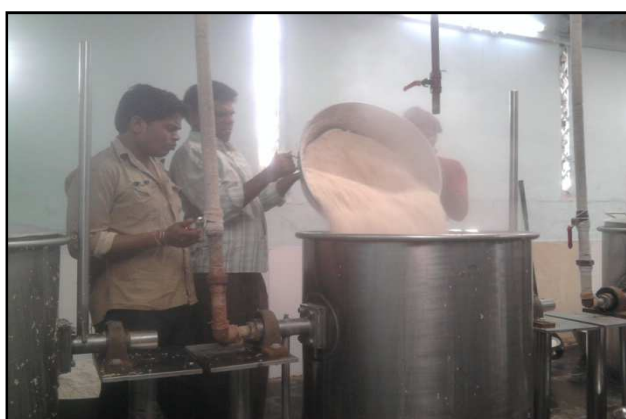
Boilers for rice cooking
